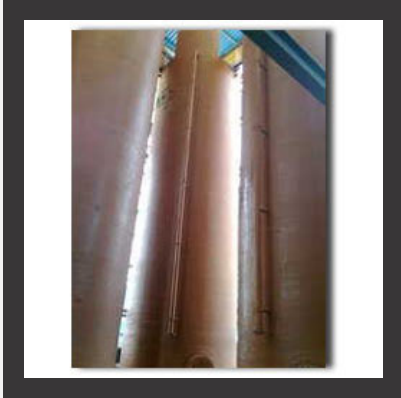
GRP Bulk Acid Storage Tank
