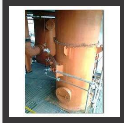
GRP Scrubbing System
