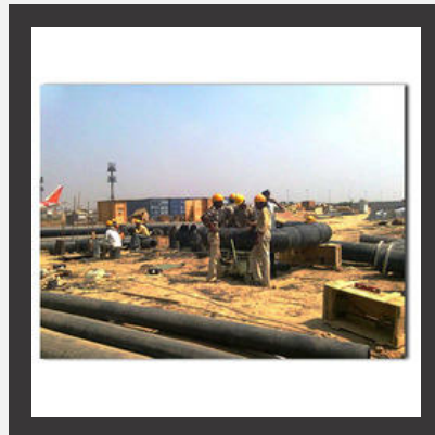
HDPE Pipe Line
