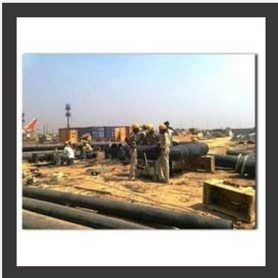
PP Pipe Line
