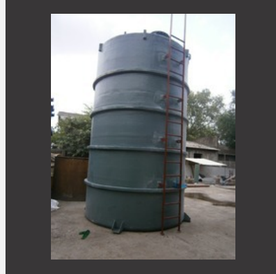
Chemical Storage Tanks
